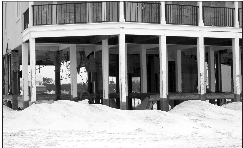
Figure 3. Successful breakaway wall performance
