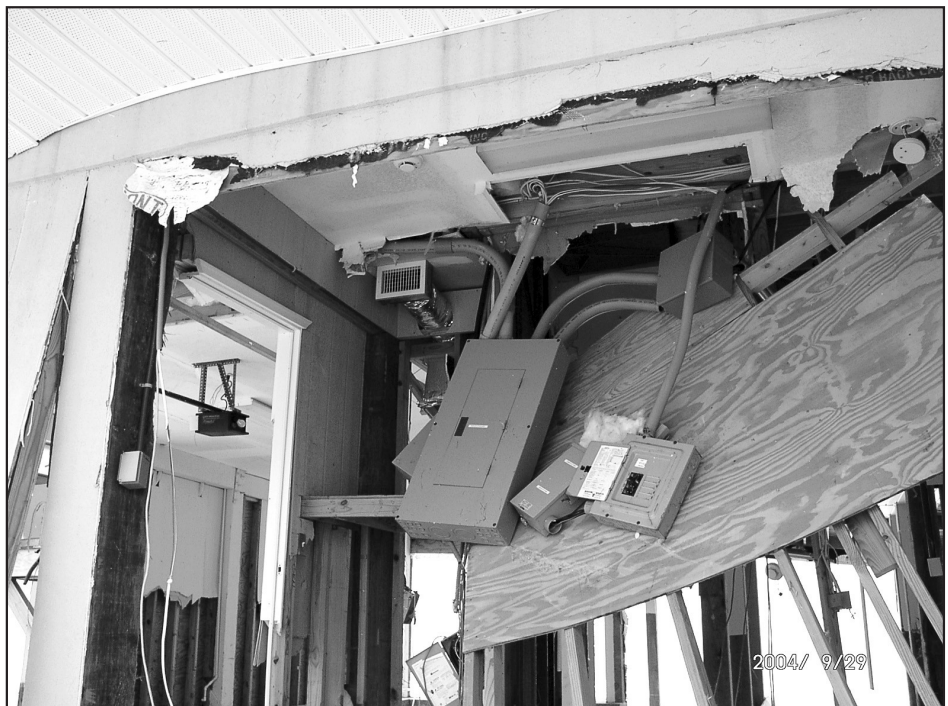
Figure 6. Non-compliant utilities attached to breakaway wall
