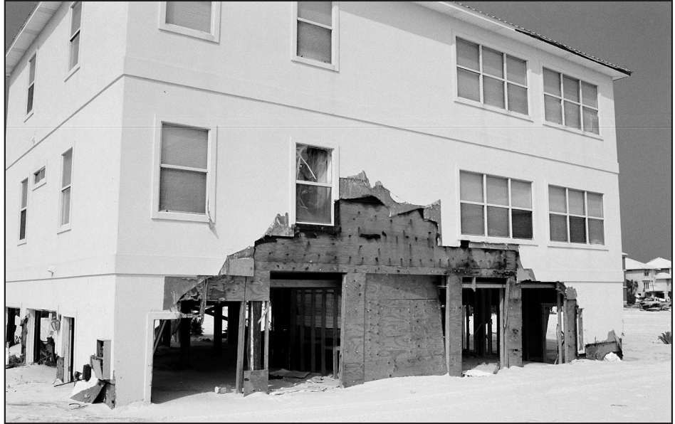
Figure 5. Non-compliant breakaway wall joint detailing
