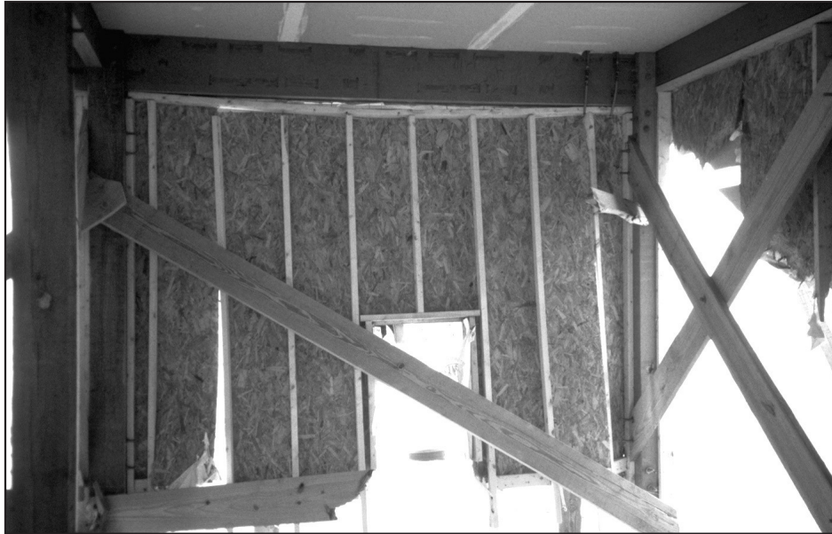
Figure 7. Non-compliant bracing arrangement
